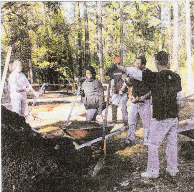
Volunteers build the new joint community garden between the North Buckhead and Brookhaven neighborhoods. Photos by Mandy LeCompte
